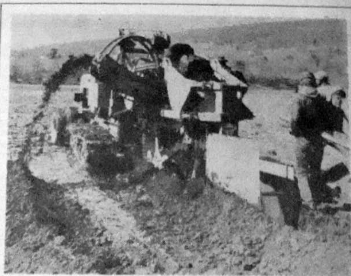
DRAINAGE TILE installation is speeded by the use of this ditching machine owned by the Potomac Valley Soil Conservation District and available for use in Pendleton County.
